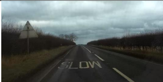
Photo 31 – Warning sign has been twisted to face wrong direction and sign appears worn
