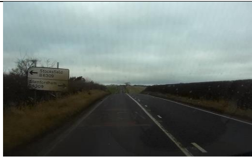
Photo 13 – Worn stack type advanced direction sign which has slipped on posts. Opportunity to improve advanced signage and provide SLOW road markings and red strips.
