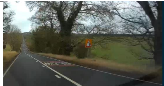
Photo 10 – Warning sign twisted to face in wrong direction and sign may benefit from an appropriate reduced speed supplementary plate
