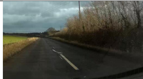
Photo 38 - Example of indistinct road markings beyond another section of road markings which have been refreshed more recently.
