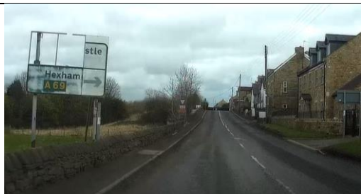
Photo 41 – Advanced stack type advanced direction sign which requires replacement and which could be re-designed to be map type showing the junction layout ahead and provided with SLOW markings and red strips.
