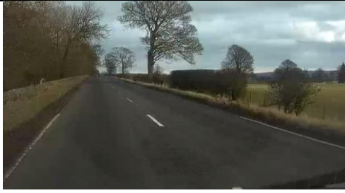
Photo 29 - Example of indistinct road markings beyond another section of road markings which have been refreshed more recently.
