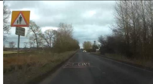
Photo 30 – Twisted supplementary plate and worn SLOW road markings and centre line road markings.
